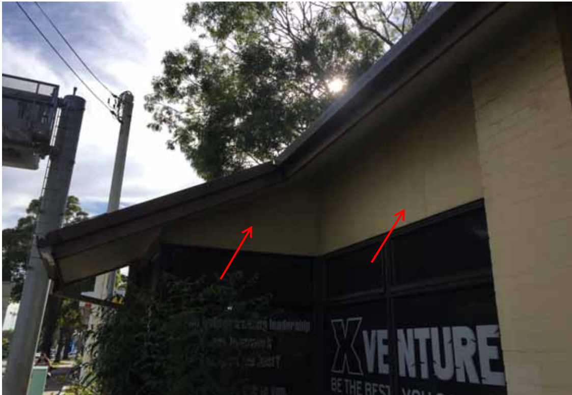
Photograph 25: Unit 2, gable and head linings (assumed asbestos).
