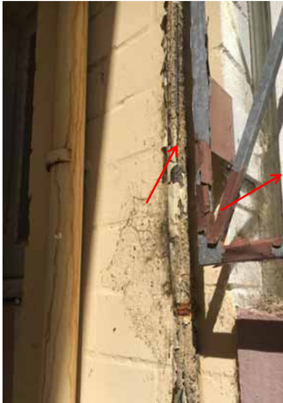
Photograph 3: Building 1, external, north facing bathroom windows, flaking white paint (lead paint).
