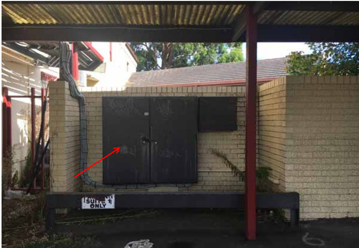
Photograph 5: Building 1, external, carport, electrical backing board x2 (assumed asbestos).
