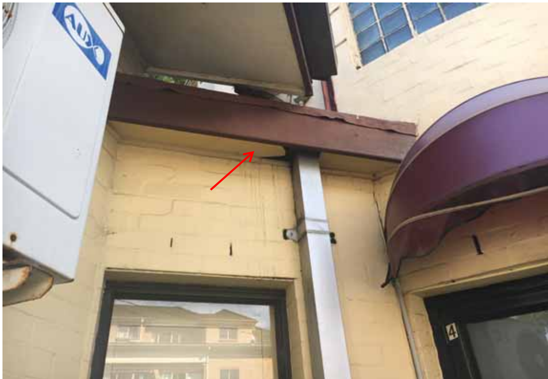
Photograph 4: Building 1, external, eaves linings near intersection with Unit 3 (asbestos).
