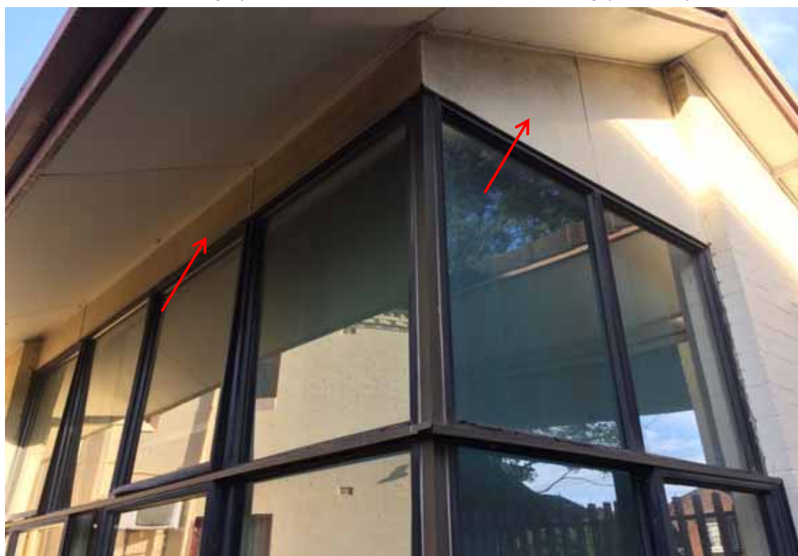
Photograph 18: Unit 3, Gable and head linings throughout (asbestos).
