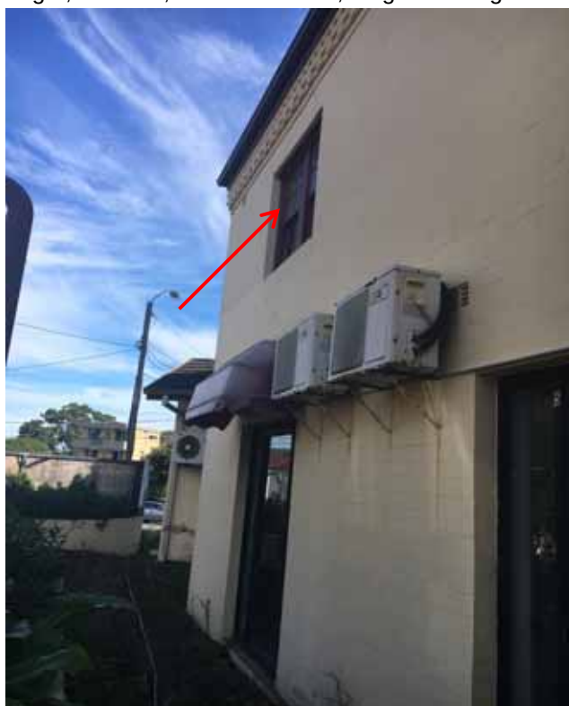
Photograph 2: Building 1, external, throughout, red paint to windows and external trims (lead paint).
