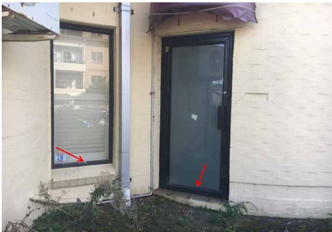
Photograph 1: Building 1, external, south elevation, beige caulking to metal windows and doors (asbestos).
