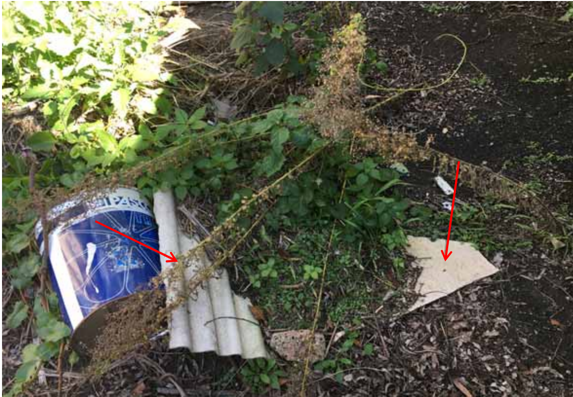
Photograph 9: Building 2, external, north-east corner of site, loose asbestos debris on ground (asbestos).
