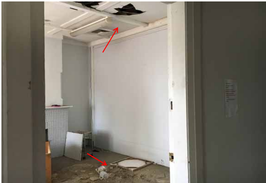
Photograph 12: Building 2, ceiling lining and associated debris, north west portion of first floor (asbestos).
