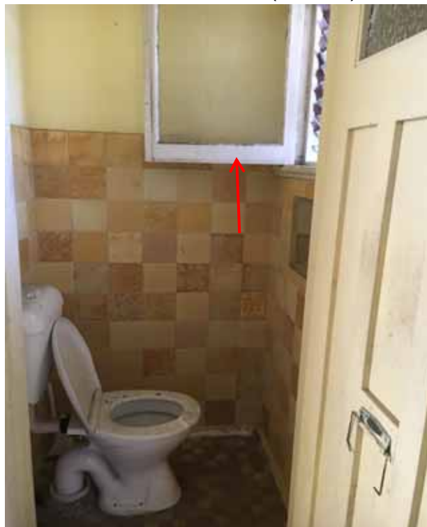
Photograph 14: Building 2, internal, white paint to window sills throughout (lead).
