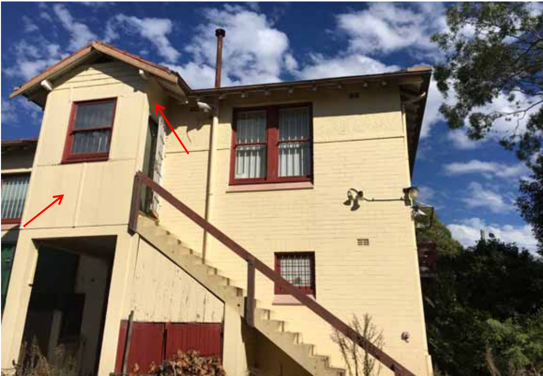
Photograph 10: Building 2, external, walls to sunroom and porch above door infill panel (asbestos).
