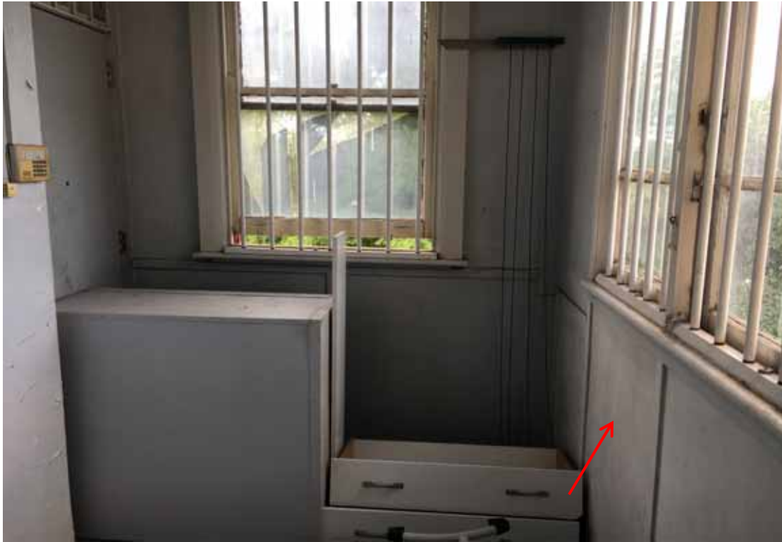
Photograph 15: Building 2, internal, sunroom wall lining, fibre cement sheet (asbestos)
