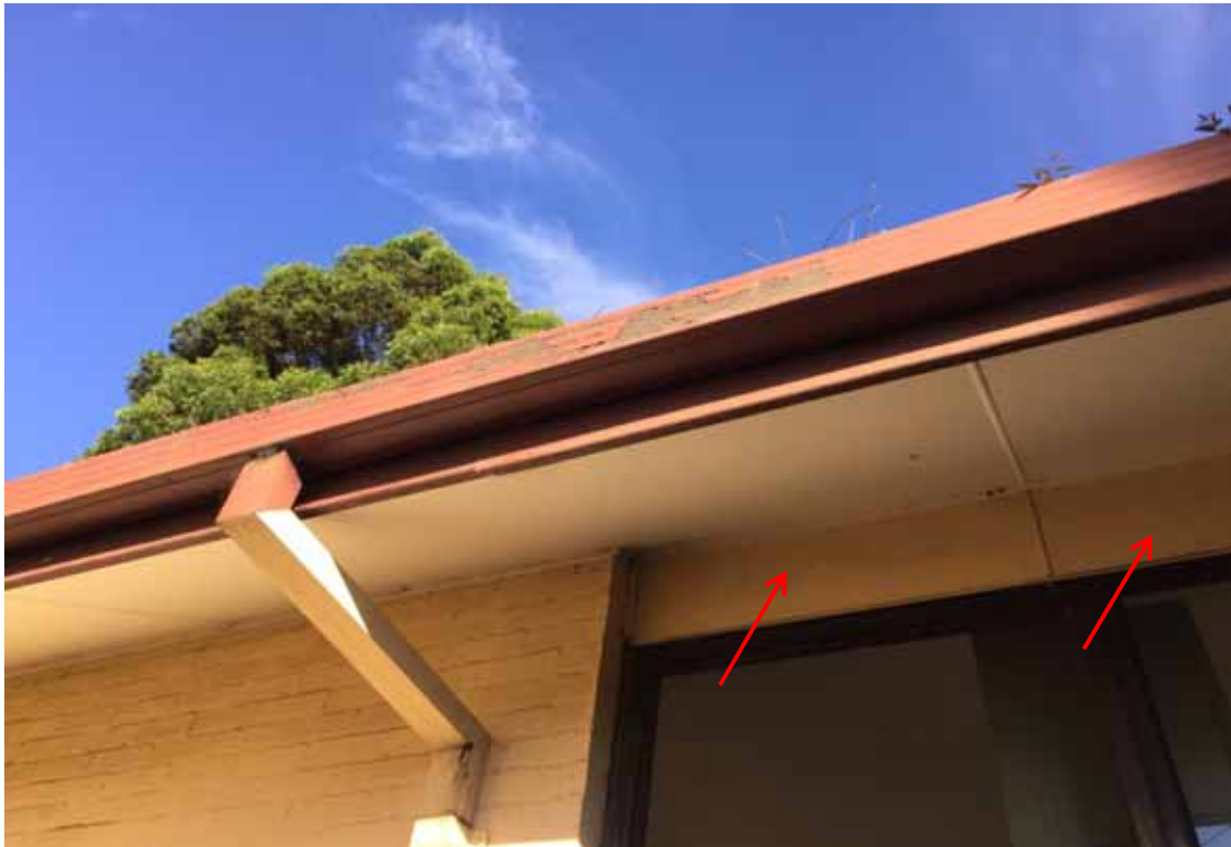
Photograph 19: Unit 3, Gable and head linings throughout (asbestos).
