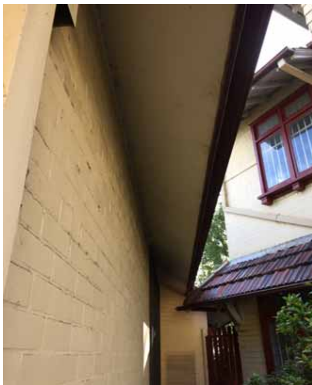
Photograph 23: Unit 2, eaves, fibre cement sheeting (asbestos).
