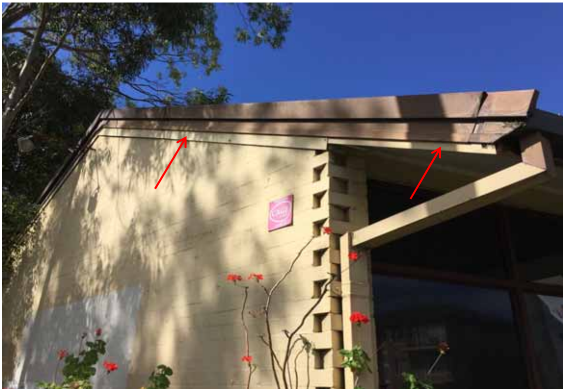
Photograph 26: Unit 2, gable ends, linings at base of metal bargeboard (assumed asbestos).
