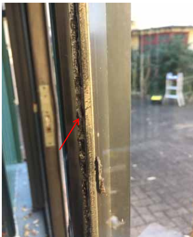
Photograph 21: Unit 3, window frames, glazing putty (asbestos).
