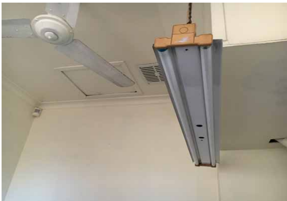
Photograph 8: Building 2, internal, capacitors in fluorescent light fittings (PCB).
