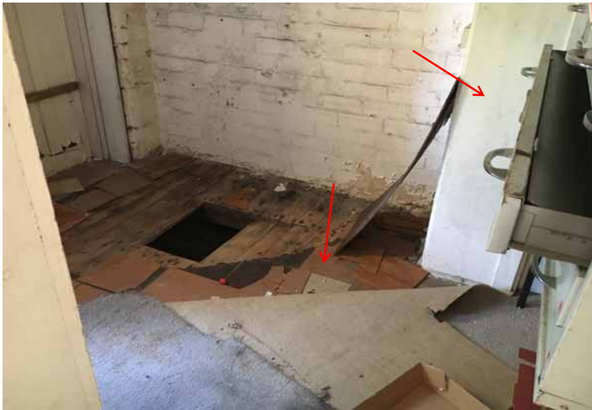
Photograph 13: Building 2, internal, rear exit room, brittle brown vinyl tiles (asbestos) and fibre cement service riser (asbestos).
