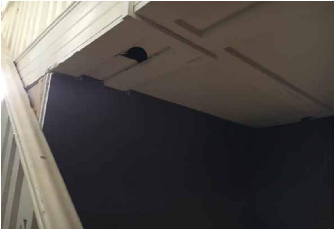
Photograph 11: Building 2, fibre cement ceiling lining below stairs (asbestos).
