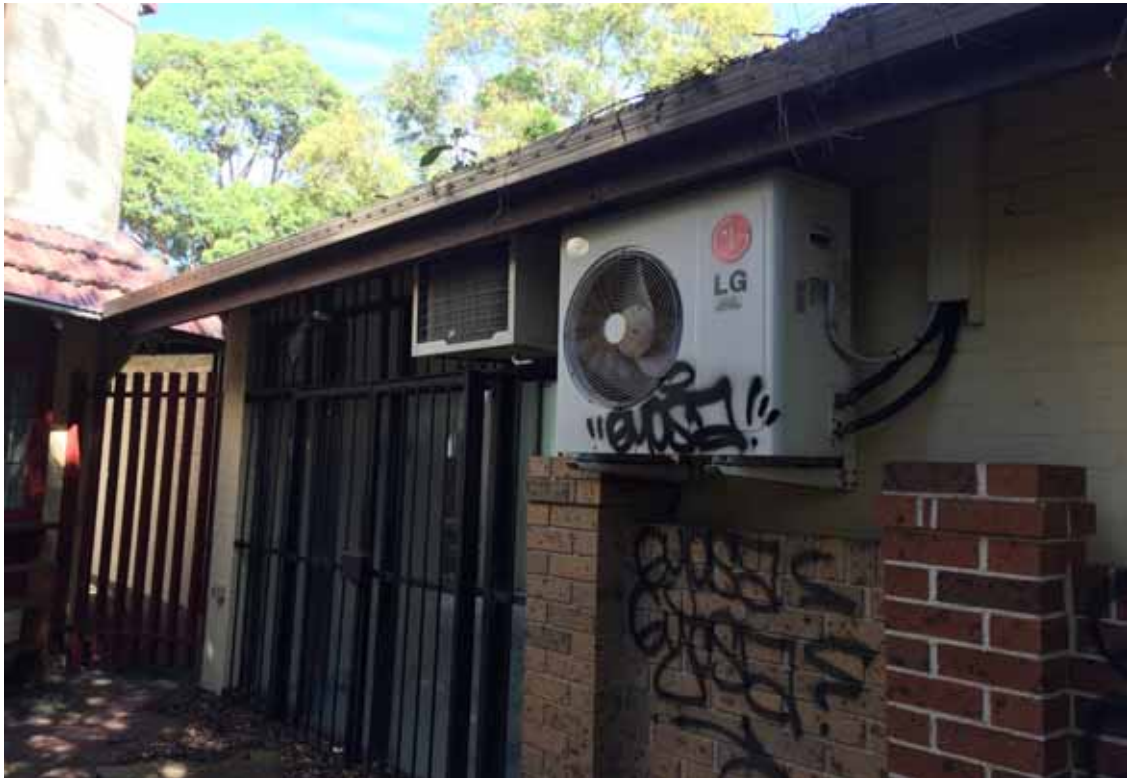
Photograph 27: Unit 2, air-conditioning units, internal insulation (assumed SMF).
