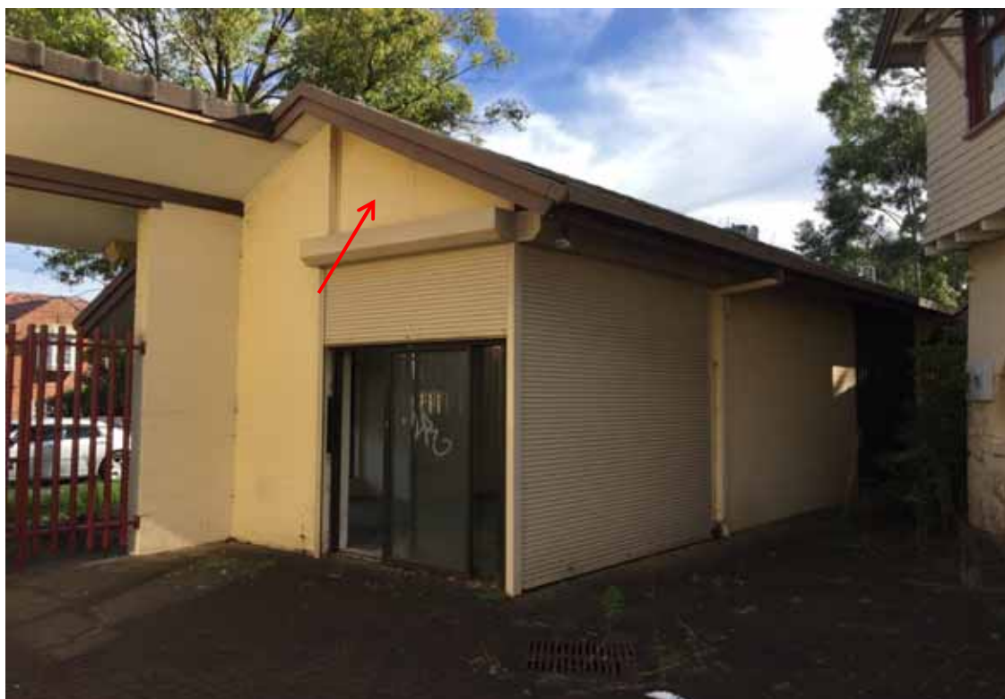
Photograph 24: Unit 2, gable and head linings (assumed asbestos).
