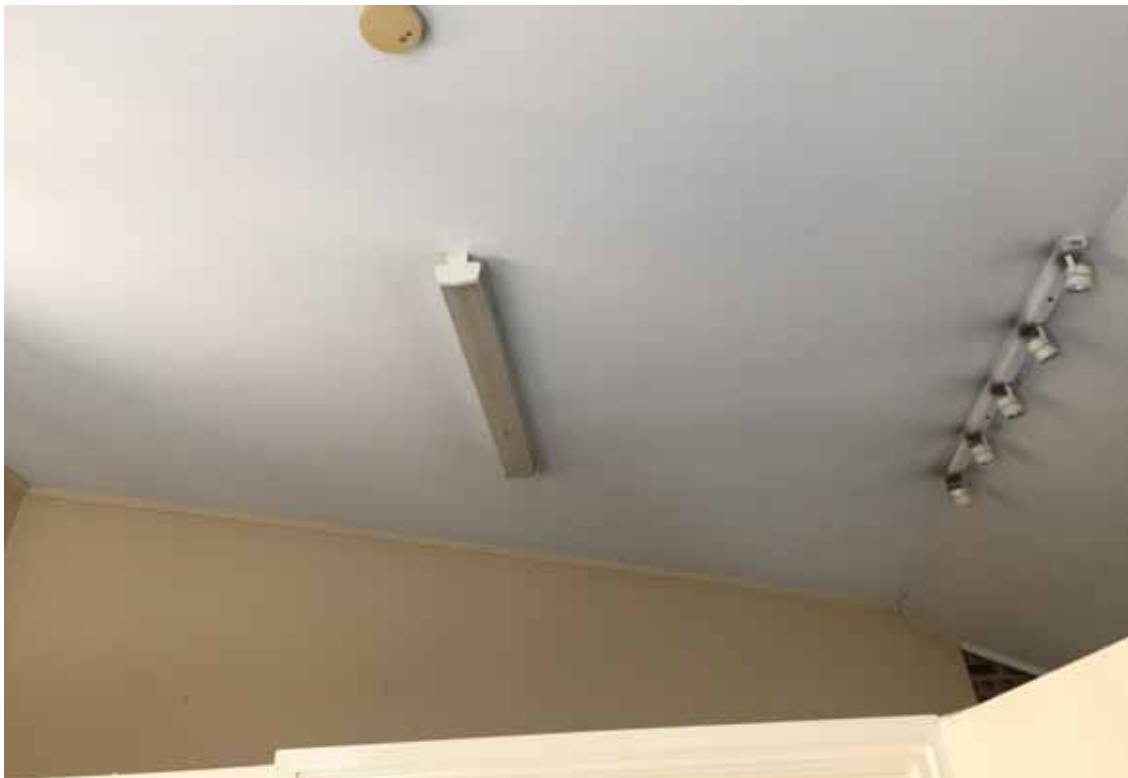
Photograph 20: Unit 3, interior, fluorescent light, capacitor (assumed PCB).
