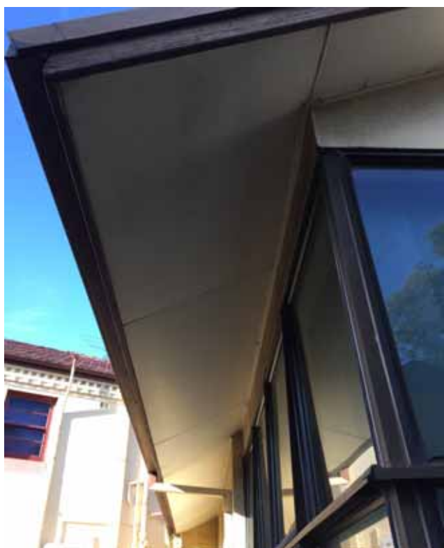
Photograph 17: Unit 3, eaves, fibre cement sheeting (asbestos).
